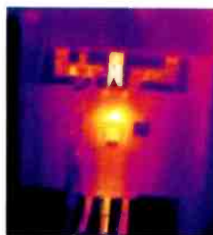
Figure 2. An example of a 600-amp disconnect switch with problems on the center phase.
