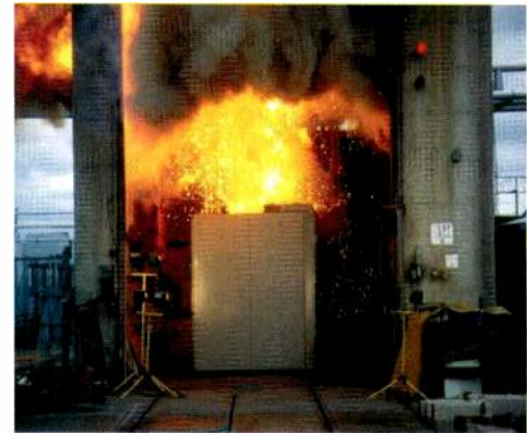
An arc flash is an electrical explosion that produces a large amount of energy. Photo courtesy EWB Engineering.
