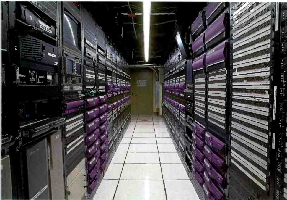
The network's IT-centric remote control and monitoring system can access thousands of individual production and distribution devices from any PC.
