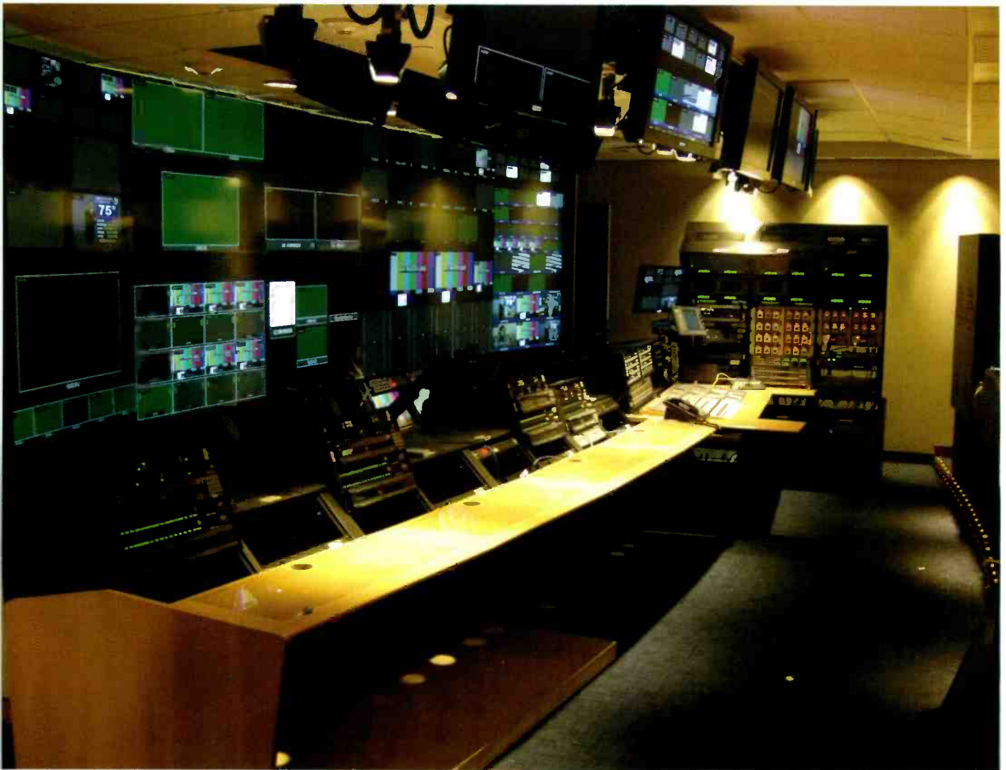
NBCU's main production control rooms monitor more than 2000 devices within the network's New York City headquarters alone.
