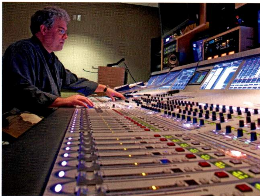
The Lawo mc 2 90 production console allows Turner Studio's Audio Control Room 22 to effectively handle the 200 channels-to-mix for "Major League Baseball on TBS" and other live shows.
