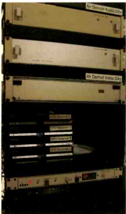
Four Samsung DTB-H260F set-top boxes are connected to audio and video distribution amplifiers.
