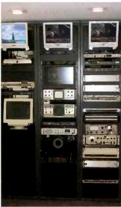
The main transmitter racks include a digital rack on the left, monitoring in the middle and analog on the right. The monitors on the top are digital off-air, analog off-air and cable.
