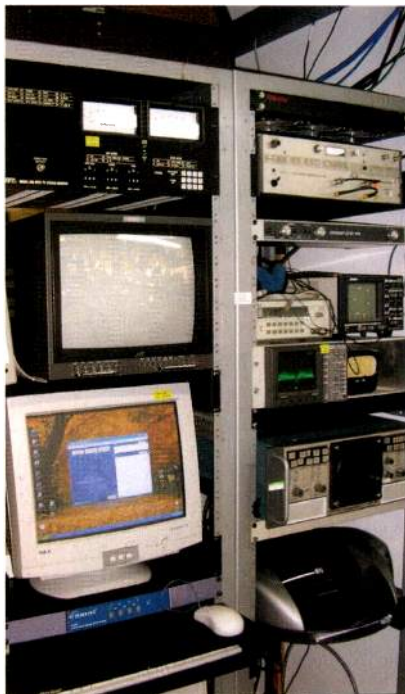
The digital transmitter and its exciter are controlled from a digital workstation that has two computers, one for system control and the other for setting up the digital exciter.
