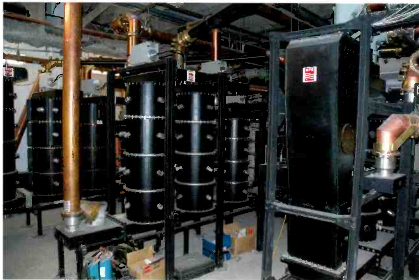
On the Sears Tower, three multiplexers were squeezed into what was previously a restroom off of what had been an old observation deck.
