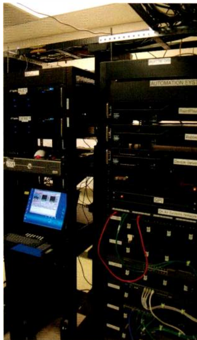
KMTP installed a Video Technics Apella video server, which is based on a gigabit network. The server can be expanded in the future as the station grows.
