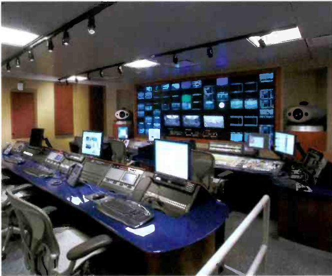
The Newseum has two identical HD control rooms with three large consoles for managing productions in the facility's two studios.
