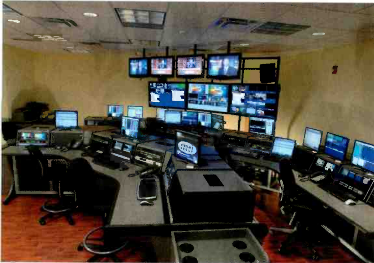
The station's new master control suite is securely linked to the old part of the building with Belden RG11 cabling, which helps to move signals back and forth.
