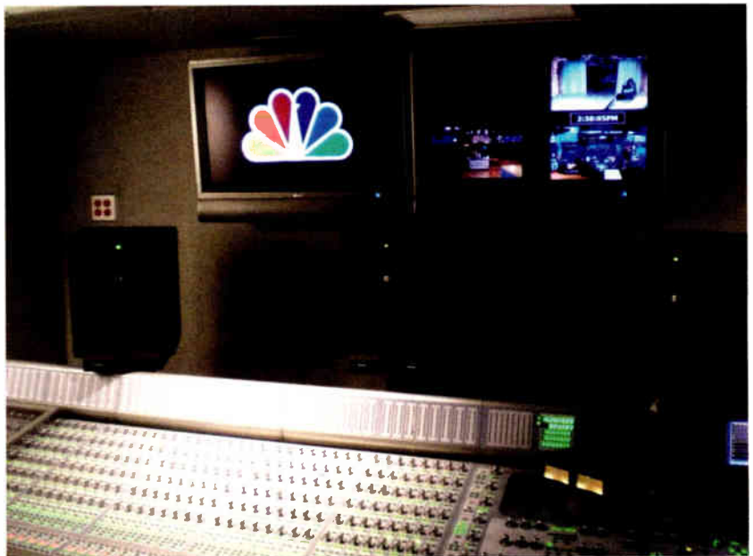
"Late Night with Jimmy Fallon" uses nearfield monitors with sound absorption at the bottom of each speaker to minimize reflections off the console.
