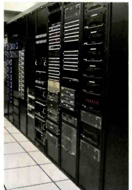
The technical operations center houses an Evertz EQX 576 x 576 HD video router.
