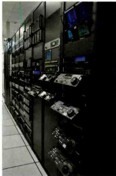
The multiformat ingest center handles the massive amount of footage that comes into the facility on a daily basis.
