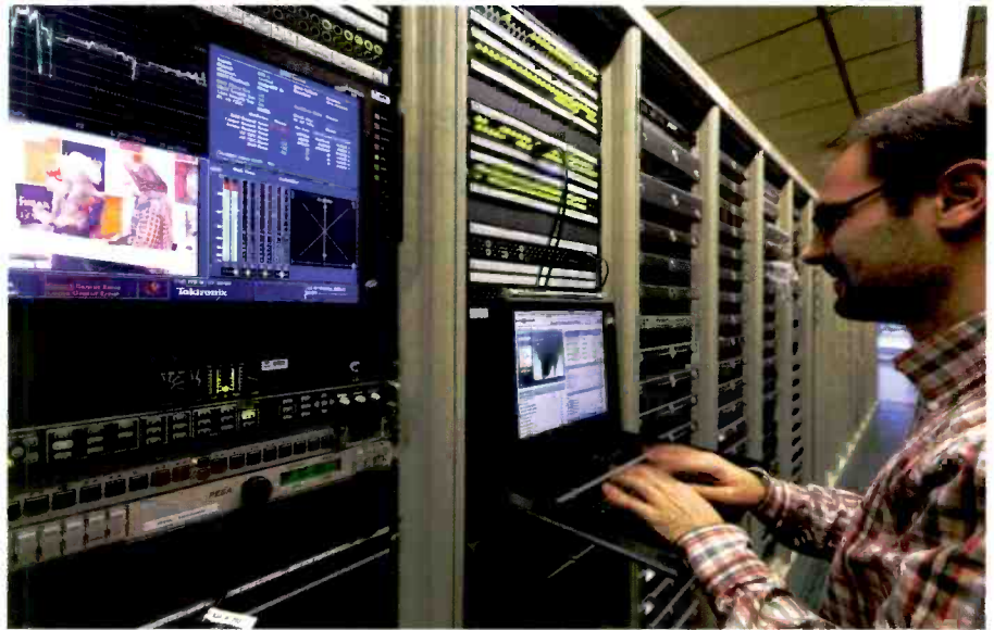
The story-centric workflow requires integration of the newsroom computer system, the MAM system, production tools, automation, archiving and the tools to manage it all.
