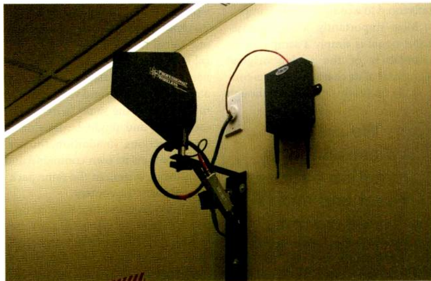
A batwing antenna provides added coverage when a subject is walking down a hallway.
