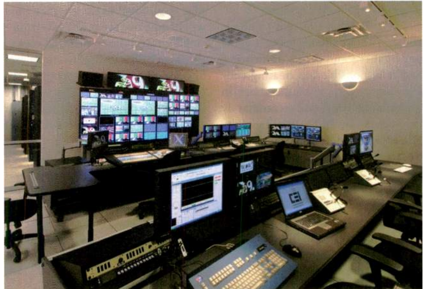
A full complement of HD technology has been installed at FedEx Field in Washington, DC, that enables the "event-day" control room to mix a variety of feeds and send images (both live and prerecorded) to fans in attendance.
