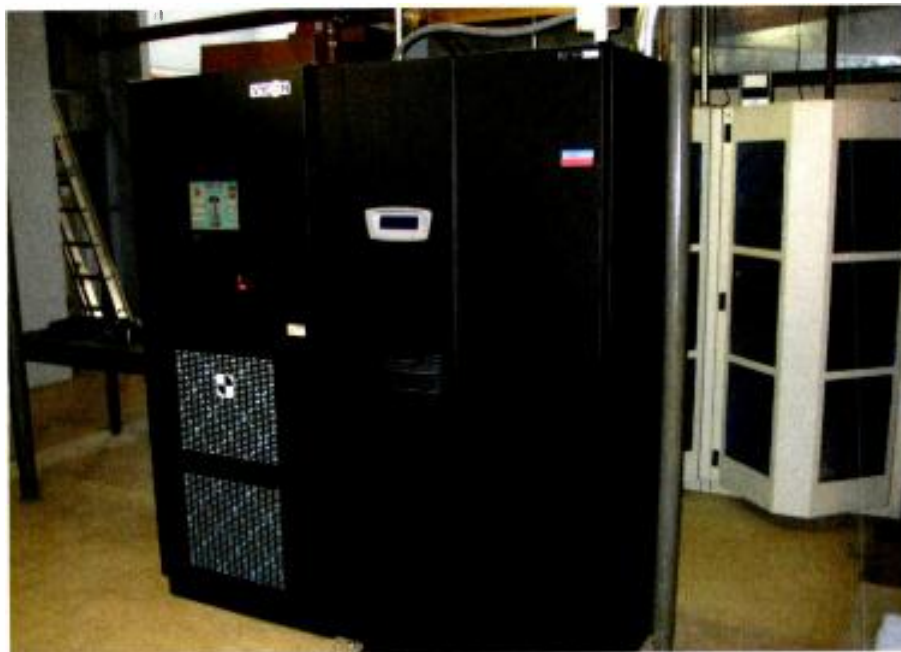
In the event of a power outage, this VYCON VDC flywheel system coupled with a battery-based UPS provides Alabama Public Television with temporary power while the station’s generator system fires up.
