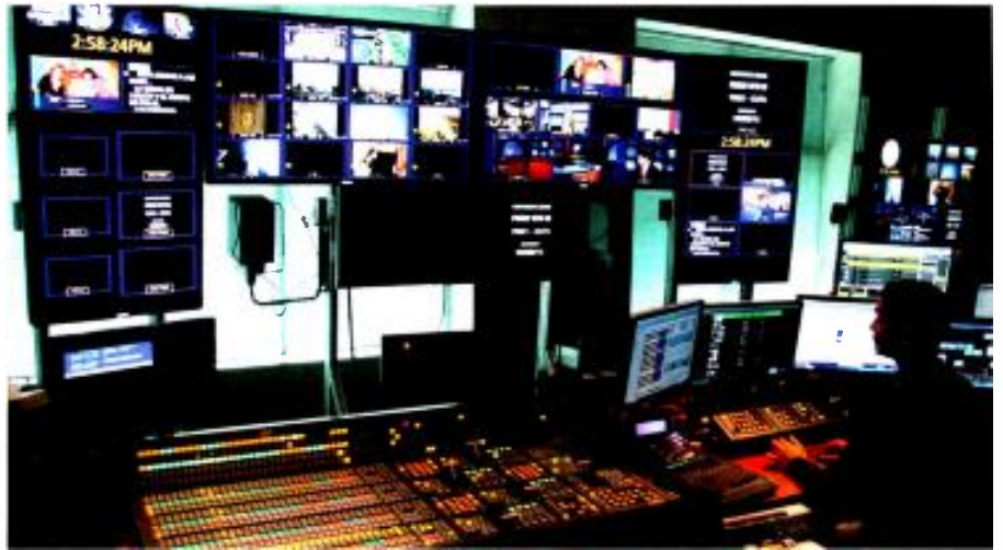
When KOMO-TV in Seattle upgraded its production facility to HD, the station added multiple flat-panel displays for monitoring. The station uses the upgraded facility to produce HD newscasts. Photo courtesy Rob Purdy.
