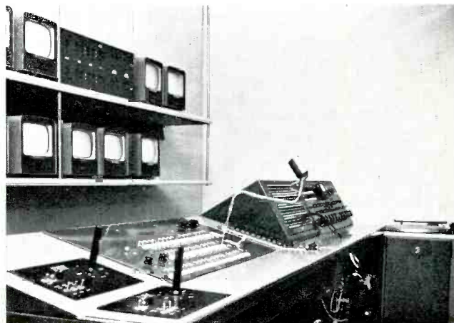
Figure 11. The subcontrol room at WKRC includes complete switching and remote control facilities.
