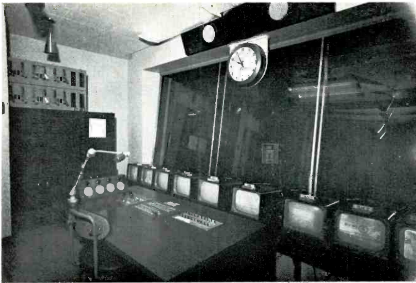
Figure 6. Video and Lighting Control Booth for Studio B showing the lighting and control panels for this studio. On the control desk can be seen the video switcher control, intercom switcher, remote control for two film projectors, two automatic slide projectors, and two RCA Video Tape Recorders. The Studio A control room is identical in physical and technical layout.
