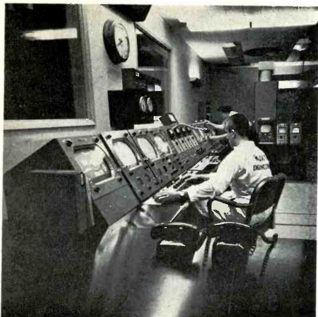
Figure 3. The Master Control room contains the microwave control for a 6-ft. parabolic antenna located 750 ft. up on the WJXT tower in addition to the preset switcher and monitors.
