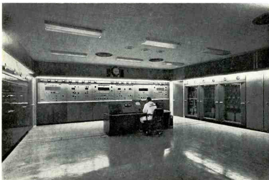
Figure 1. Transmitter room of WJXT. Across the back is the main 35 KW transmitter. On the left side is the 5 KW auxiliary transmitter. A 10 KW FM transmitter is on the right. All transmitters are controlled from the engineer's control desk.
