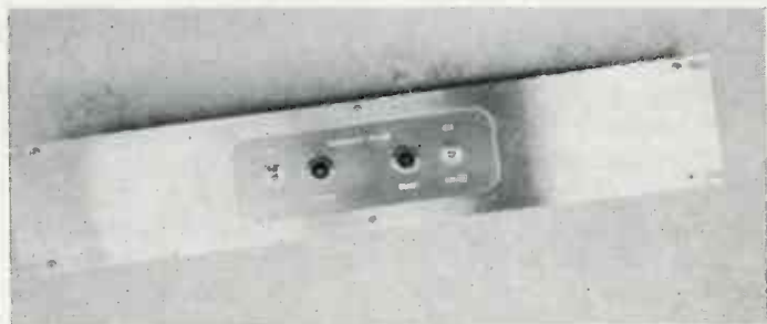
Figure 5. Operator's eye view of the alarm unit in the control room.
