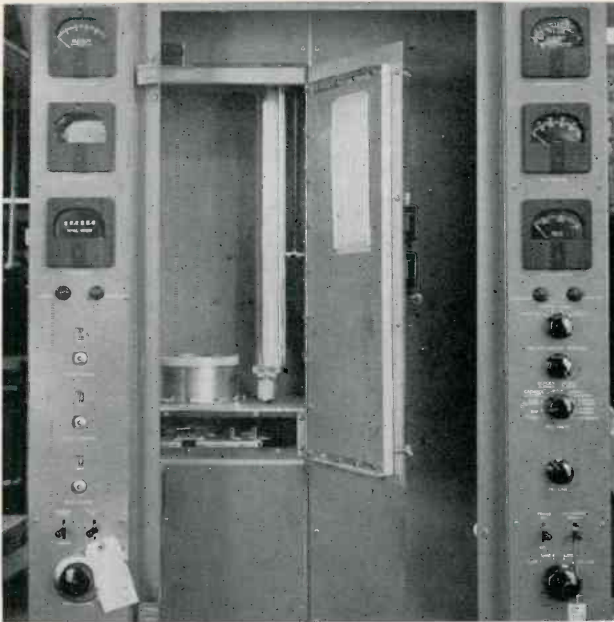
Figure 3—Front view of the 10 kw PA showing RF cavity.
