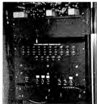
Fig. 6. The remote control unit installed at the WDCX (FM) transmitter location.
