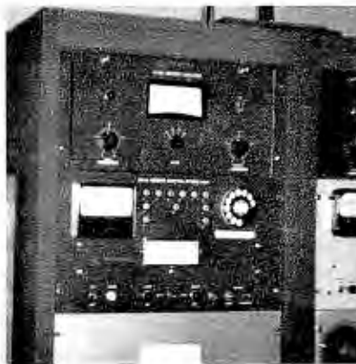
Fig. 5. ITA remote control unit installed at the WDCX (FM) main studio location.
