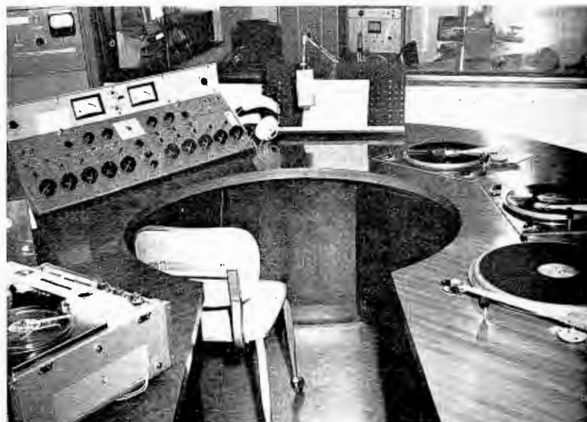
Fig. 2. Completed console desk with all equipment installed.
