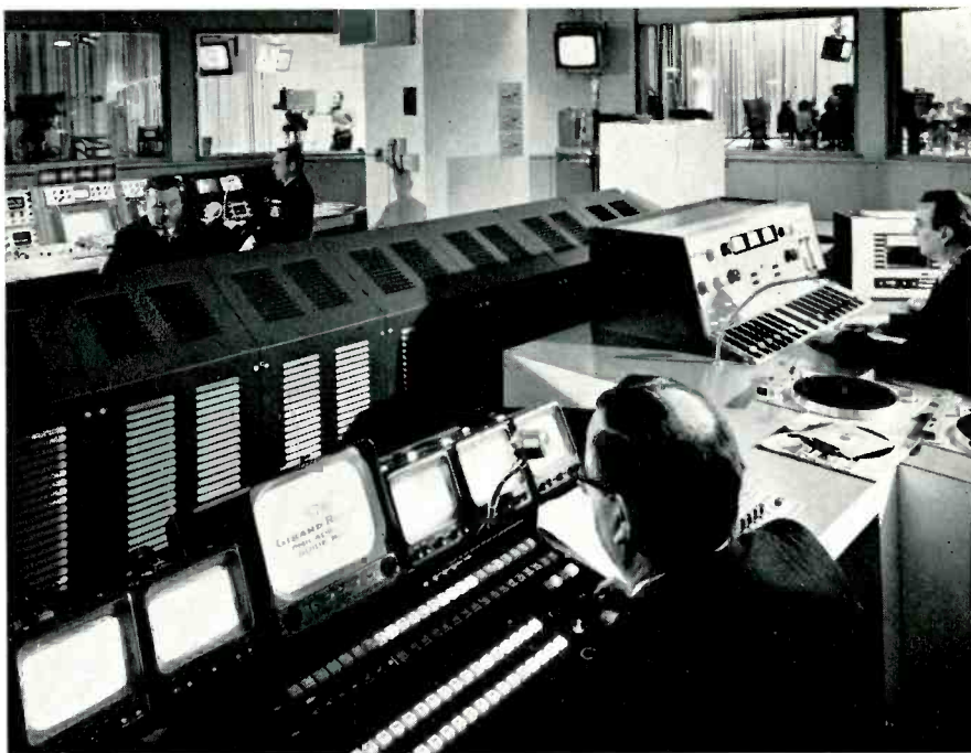
Fig. 4. Television master control, located adjacent to studios at third floor center.
