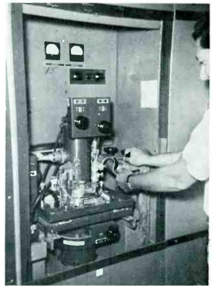
A regular program of tightening high current and RF connectors is wise.
