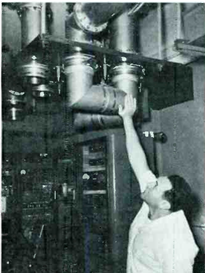
A "feel test" may be used to locate trouble in transmitter RF plumbing.
