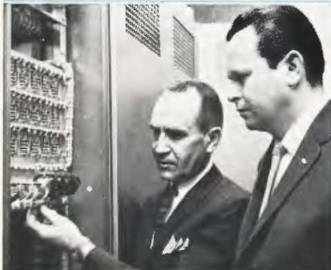
The control center of WOR-AM-FM is wired with Belden 8451 and 8700 miniature broadcast and audio cables. Explaining the complexity of the installation to George Kyros is Orville J. Sather, Director of Engineering for WOR-AM-FM.
