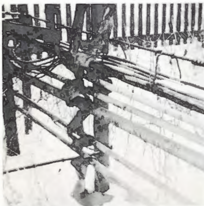
Because of line expansion and contraction, strap had to be replaced.
