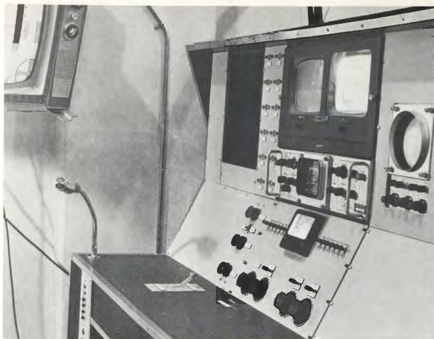
Fig. 4. Delegate switcher controls inputs to KCSM-TV channel-14 transmitter.
