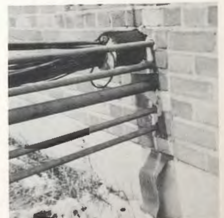
Watch for breaks in the ground strap where it enters transmitter building.
