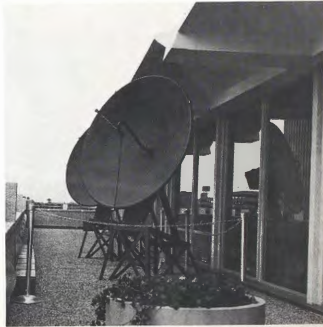
Fig. 3. Main and alternate transmitters of WTIC-TV STL.
