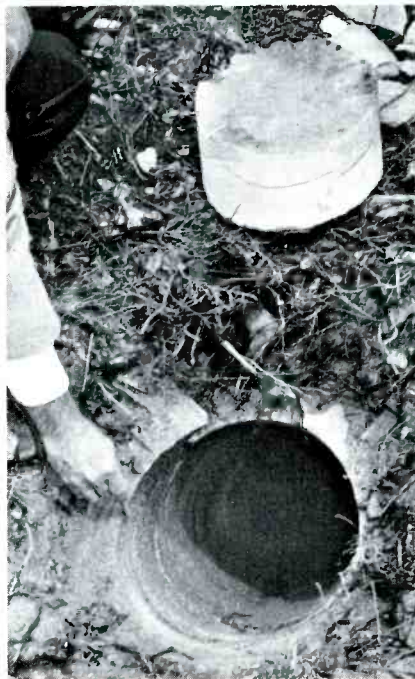
One of the 12-inch wide anchor holes and another short core of fractured stone.
