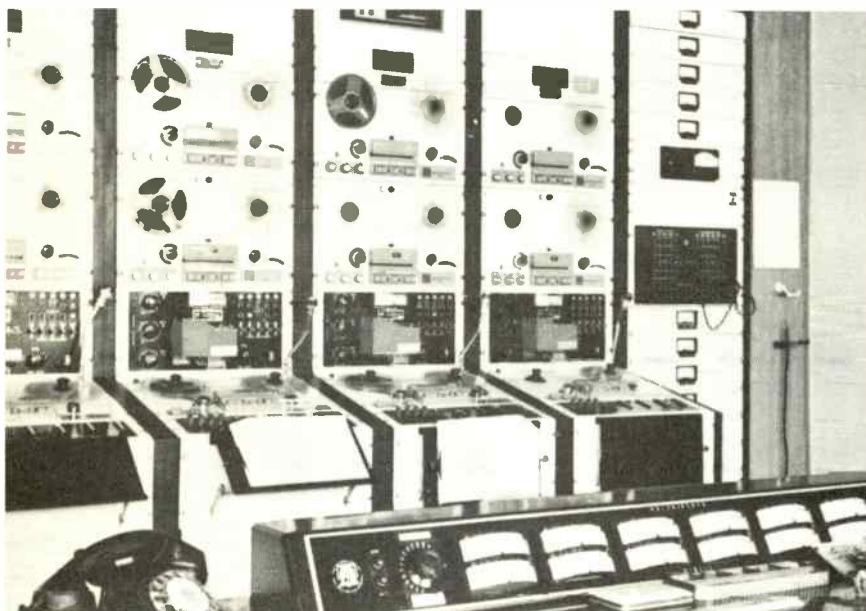
Fig. 1 Master control system has all but eliminated jack fields. The only one left is shown at far right in foreground and is for metering of all transmitter feed lines.
