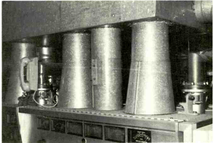
Ductwork in an air cooled system used on a UHF transmitter.
