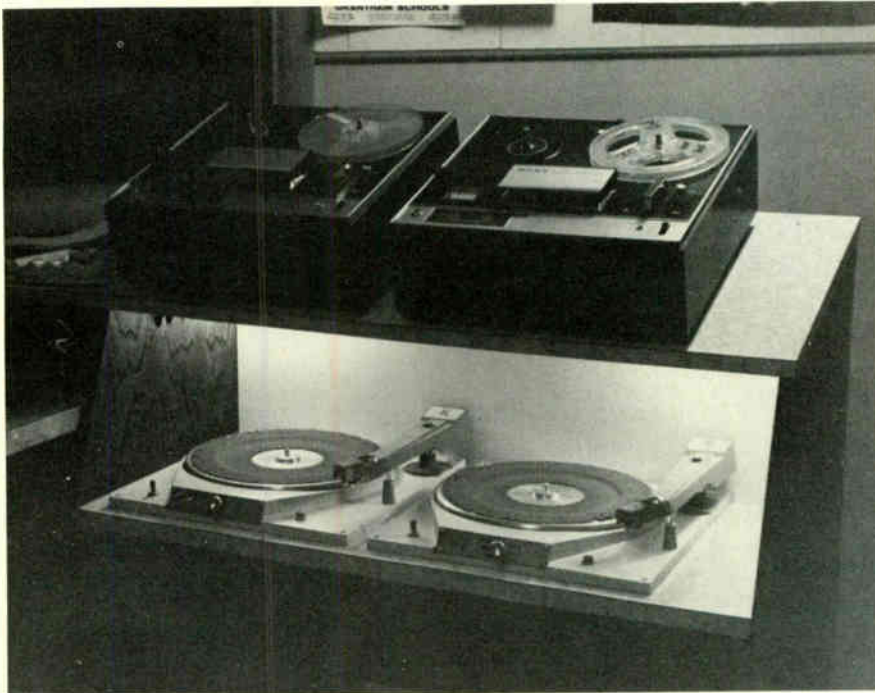
Fig. 5 Back lighting protects turntables and allows lower than usual control room light levels.
