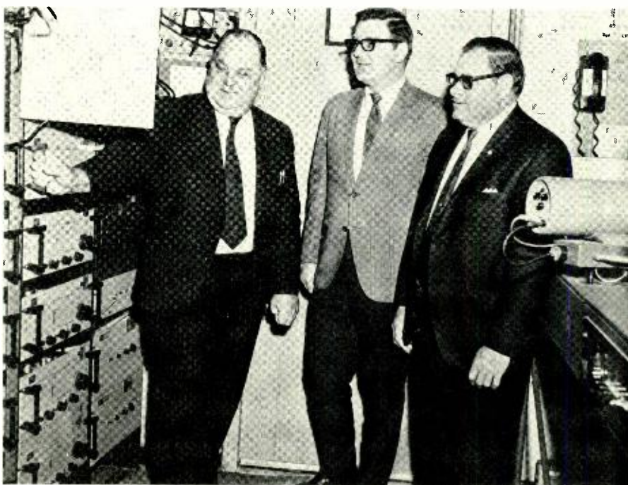
An emergency warning system has been installed in the Streator TV Cable Co., Streator Ill. The Civil Defense and Police warning system is reviewed by Leo Wilkinson, Wib Beckendorf and Mayor Lux.
