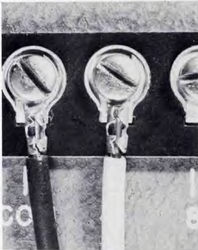
Fig. 1 The terminal connectors shown here are crimped to the wires. This is an especially hazardous practice if the wires are copper. Creeping corrosion inside the clamp is possible.
