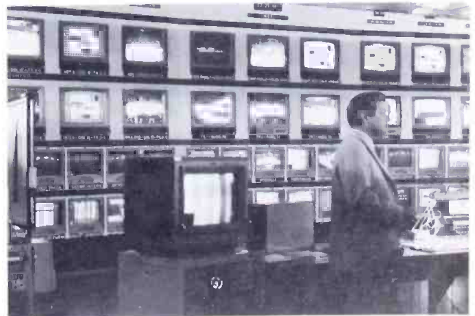
Central switching room at DOZ center provided constant checking on inputs from venues. Labeled by venue along venue along the bottom two rows and by destination on the top two rows.
