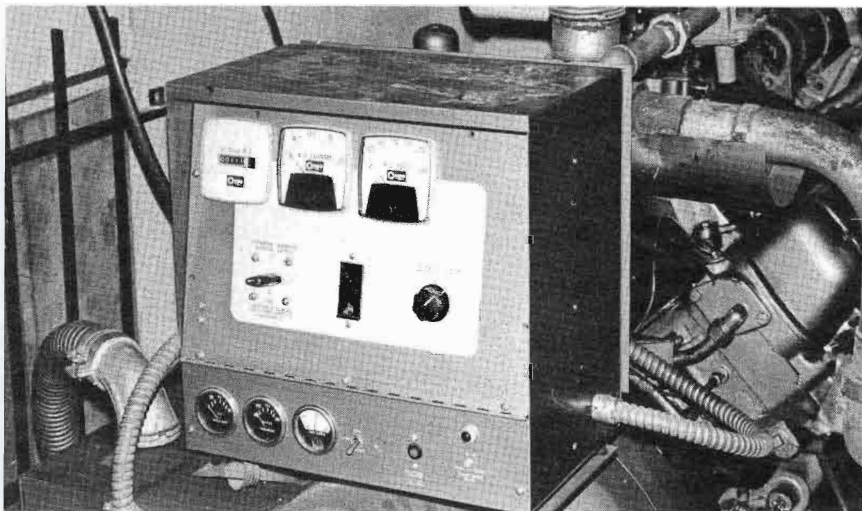
Fig. 3 Operation of the 50,000 Watt generator is completely automatic. Failure of any one of three phases of the commercial power will start the unit. When the power returns to normal, the generator will continue to run for about five minutes and then shut down. (Note the security bars over the air intake at left.)
