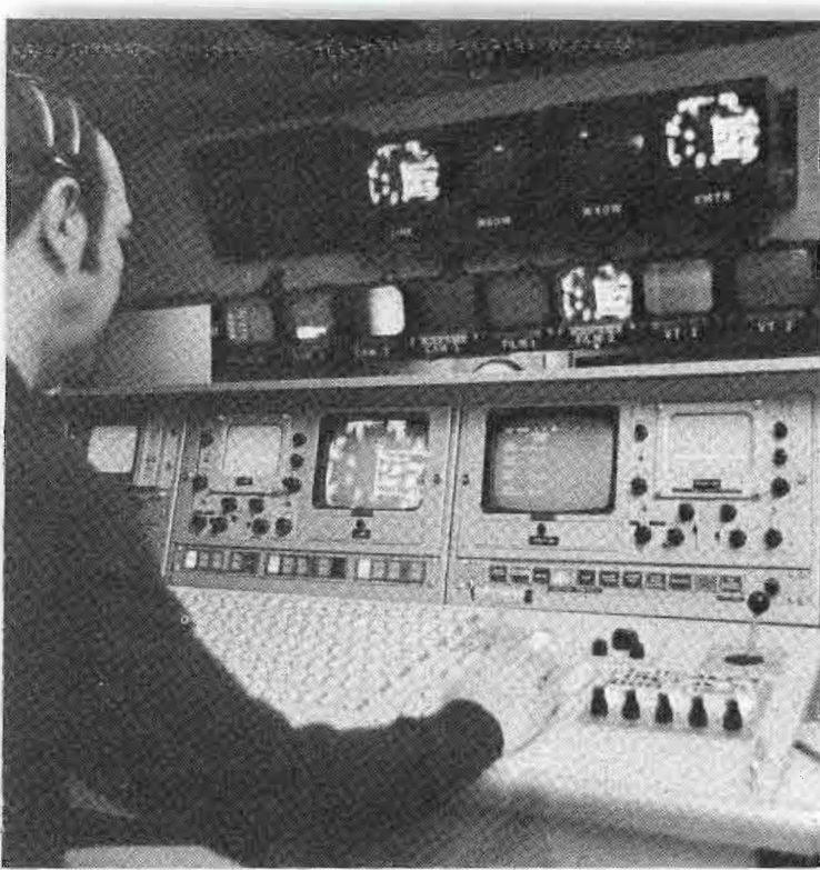
Engineer Homer Bellus is shown here switching a station break. The LINE and XMTR monitors show the WKOW-TV ID being aired, while the ID logic has switched black to WAOW and WXOW-TV.
