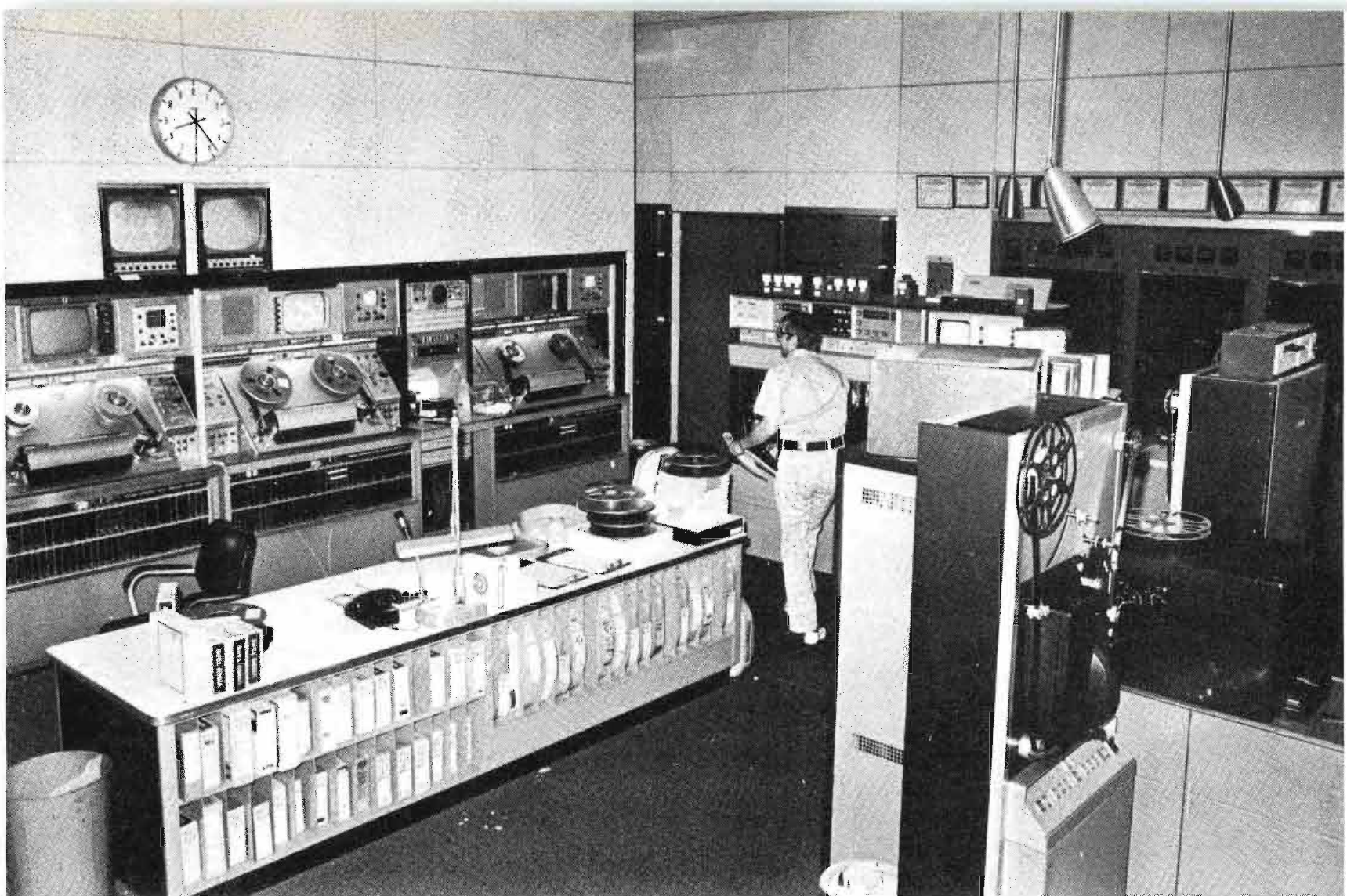
Fig. 3 In the WIIC-TV control room, computer read-out monitors are mounted above the VTR's. In the film chain area, they are suspended from the ceiling. Chief Engineer Bob Wehrman also has a monitor in his office so he can keep tabs on control room operations without being there.
