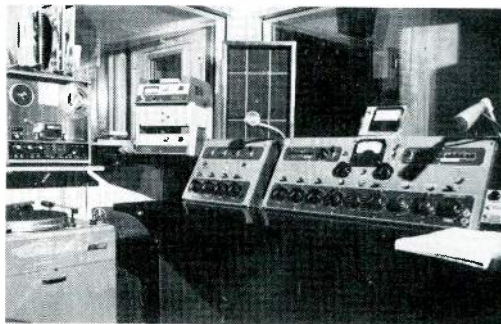
This is the audio end of the KMJ-TV control room as it looked before installing the new console and extender panel.
