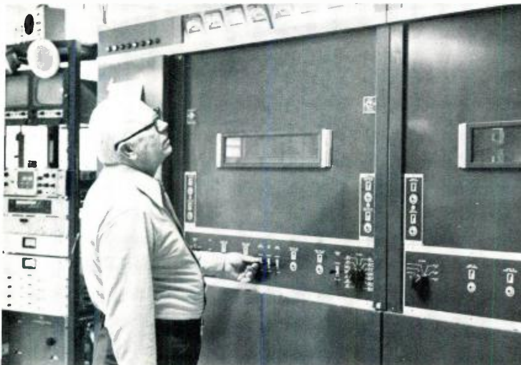
Once inside the Court House Plaza Building, KSFY-TV engineer Clarence Ausham checked the controls of the temporary lashup.
