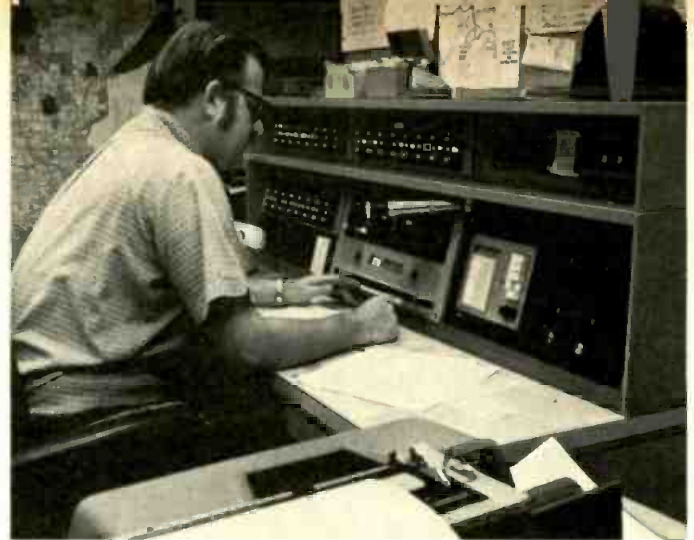
The specially designed master control console is the core of the communication system. More than 40 channels are covered, including communications with two-way equipped radio cars.
