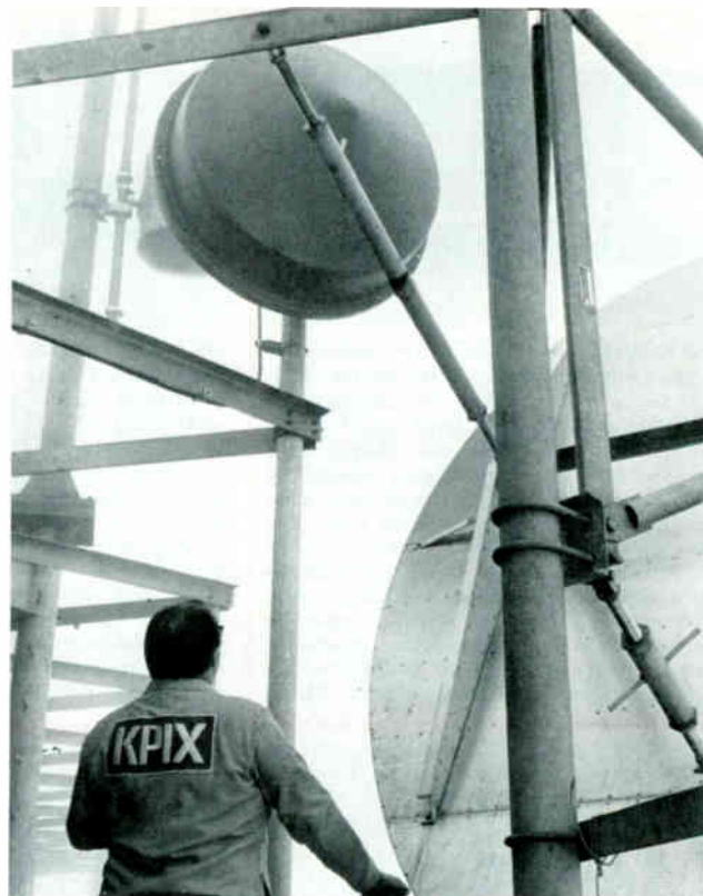
Figure 5. Protected dish on the 2nd level, some 1020 feet above sea level, receives 13-GHz signals from Mt. San Bruno. Passive reflector on right is from some other service.
