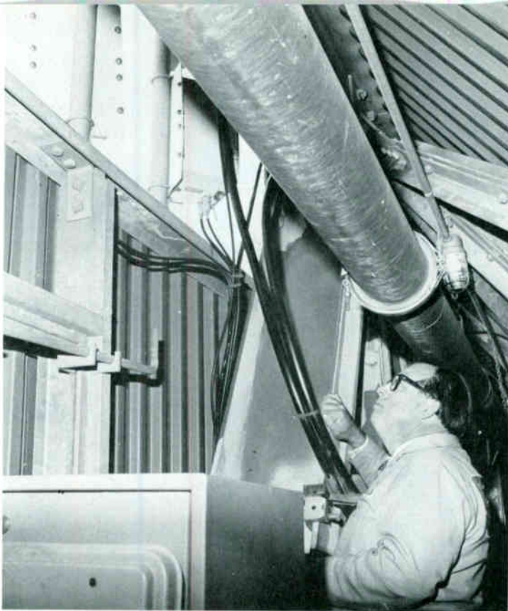
Figure 3. Nurad ENG pickup horns are mounted on the 4th level. Catwalks are sheltered up through the 4th level to protect equipment and permit all-weather access. Specific antennas are selected by remote control from the downtown ENG control point. Signal is down-converted to 70 MHz IF and piped down to equipment room over coaxial cable, as with point-to-point links.
