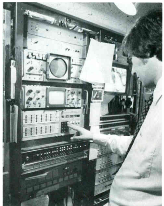
Figure 7. Charles Rose, KPIX studio technical supervisor, examines the remote control unit in downtown studio master control room. Unit enables any of 26 communications functions to be dialed up remotely, allowing picture quality, waveforms and other functions to be inspected.
