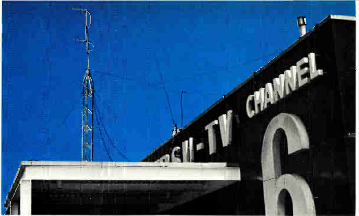
Fig. 1 The 462.55 MHz CB antennas for communications between AM-FM-TV studios and the AM transmitter site.
