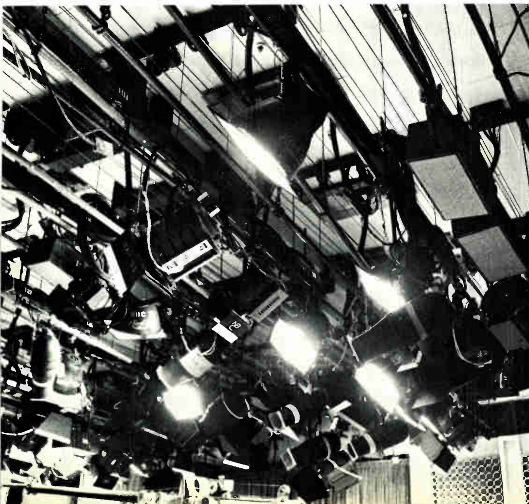
Fig. 2 Here are some of the 325 fixtures. All are connected overhead in wireways and run into the floor above the studio.
