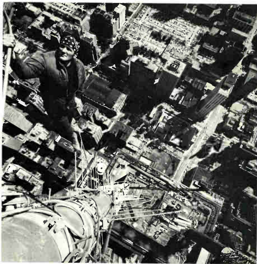
Nearly 1,400 feet above Chicago streets, on a TV broadcast tower atop the 100-story John Hancock Center, an ironworker checks one of the six television antennas installed there. Four of the six TV stations began broadcasting from the new site after Jonas Dovydenas, fearless Chicago photographer, climbed near the top of the 349-foot tower to get this dramatic picture.
