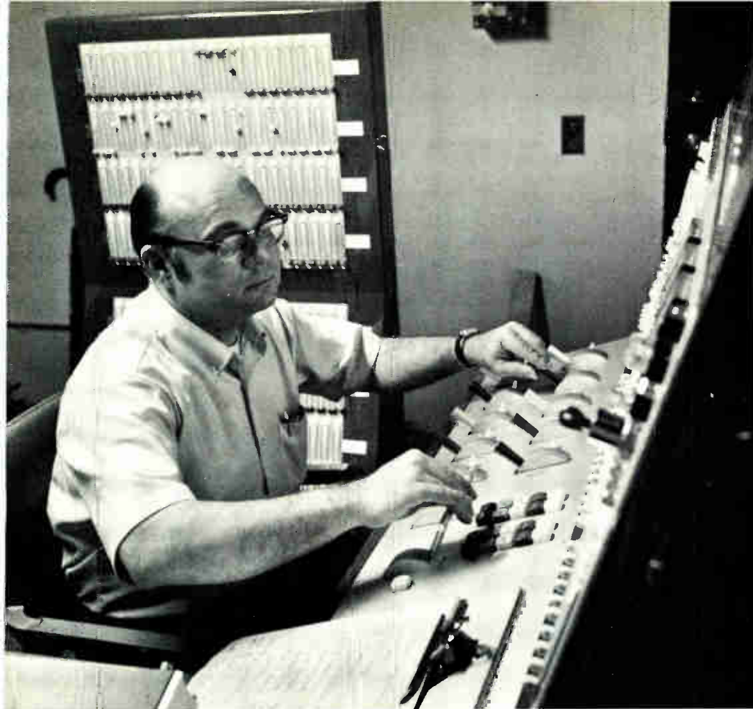
Fig. 1 Jerry Savitch at the master control console which provides for sub-mastering and blink-free cross fading. The system has 42 dimmer circuits, 18 non-dim circuits, connecting approximately 325 fixtures.
