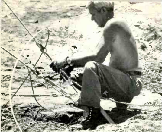
Top two tower sections are ready to be raised, with three tower-guy assemblies in place.
