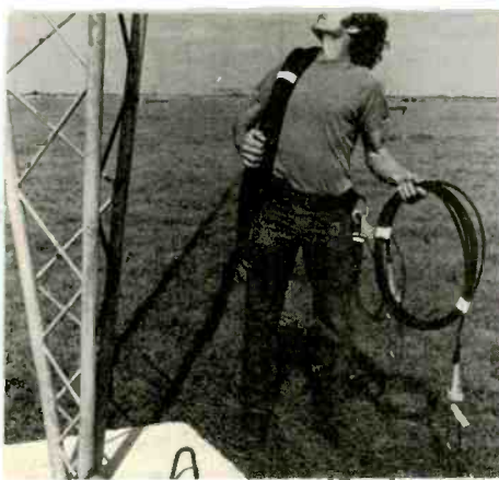
Rigger inspects tower in preparation for installing Kevlar aramid fiber guy stabilizers.
