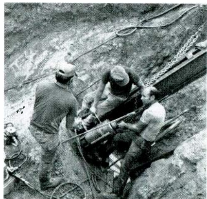
Construction workers prepare to proof load—one of five anchor cores at Anchor C-2.
