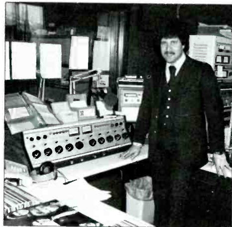
LPB S-20, 10 mixer dual stereo Signature II audio console installed in WGLU air studio.
