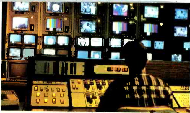
The Master Control Room line monitor racks with switcher control.
