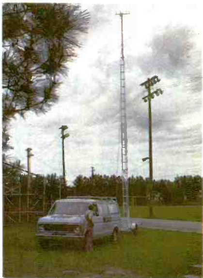
A second winch is used to raise the inside tower section for maximum height.
