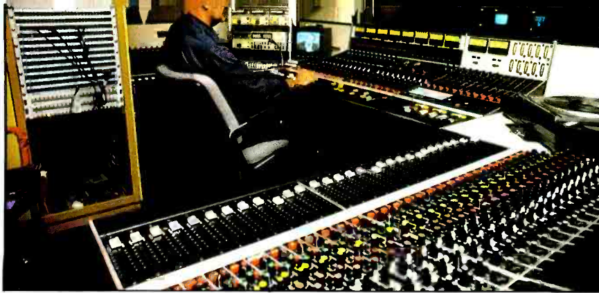
The recent installation of an M-series console from Ward-Beck in the KPIX studios, San Francisco, enhances audio operations for production and on-air. Peter Glamona, engineer, is at the controls.
