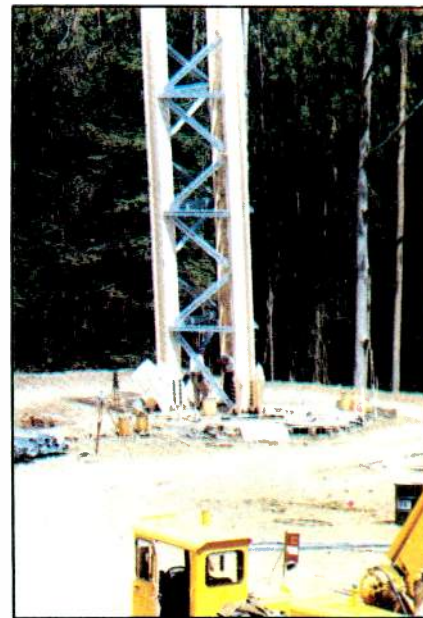
First section of north tower leg is in place. Note crane in foreground. Transit is used to check angle; men in background show scale of leg. (Aug. 30, 1971)
