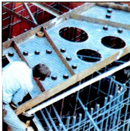
Pattern-plate supports giant "J" bolts that will attach to base leg of tower. Bolts are as thick as a man's wrist (April 6, 1971)
