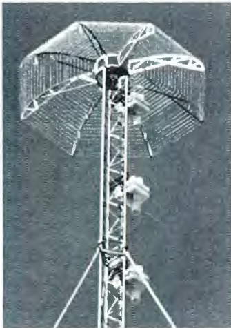
LEA LIGHTNING BARRIER. Typical Hemispherical Dissipation Array in use of a broadcast site.
