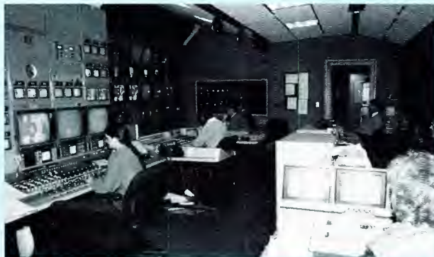
CBS Control Room 41 features the latest equipment available.
