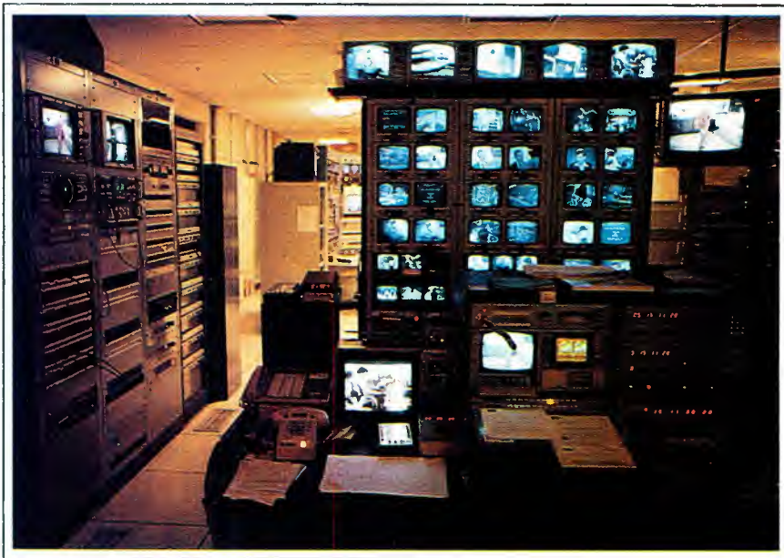
(A) The automatic commercial insertion center is just visible beyond the left side of the Warner-Amex master control center area.
