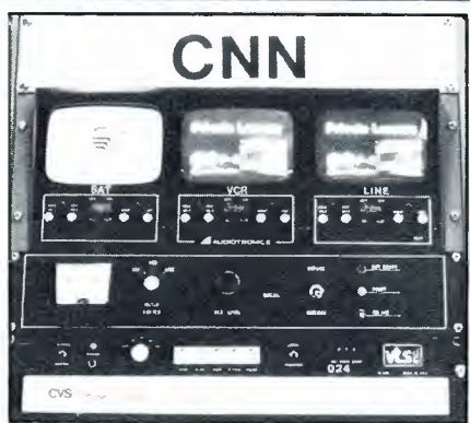
(C) Equipment (at left) for one channel includes video monitors for satellite, VCR and line; the status panel, with audio metering and selection switch; the automatic commercial insertion unit; and the time base correction unit.
