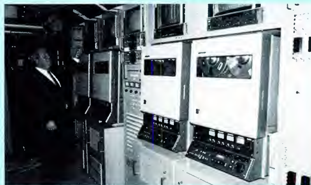
Shown are a few of the 350 racks of equipment in the CBS Broadcast Center, which support production and keep CBS on the air.
