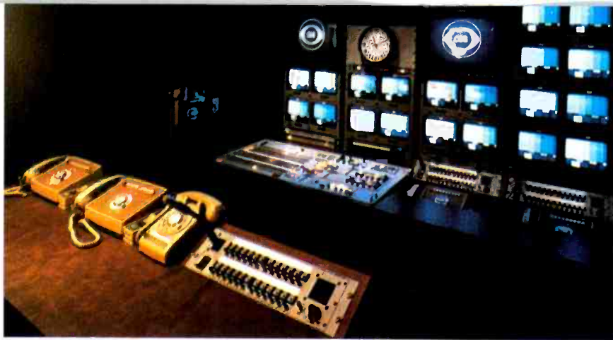
The production area of the truck contains 26 monitors, video switching and positions for the director and producer.
