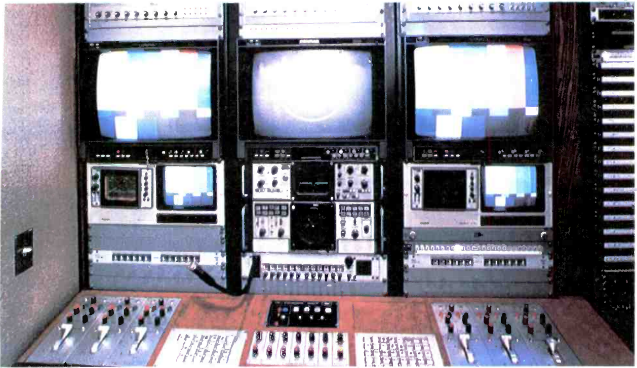
The video operator area provides controls for up to six hand-held cameras, along with monitoring and ancillary equipment for video, as well as microwave transmitter/receiver and antenna controls.
