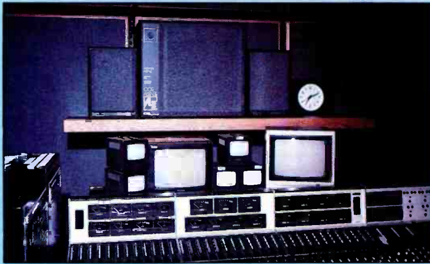
Mounted on a shelf above the Ward-Beck audio console is a pair of Sentry 100A loudspeakers and a larger size Sentry 500 between them.
