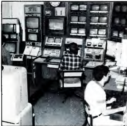
KTHI's master control room is shown as it is today. An American Data 3111 switcher is the heart of the system.
