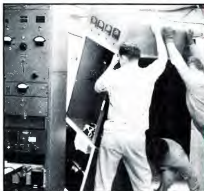
Transmitter installation work is done at KNDO-TV in preparation for station sign-on. The UHF transmitter is an RCA model, as are the frequency and modulation monitors on the left.
