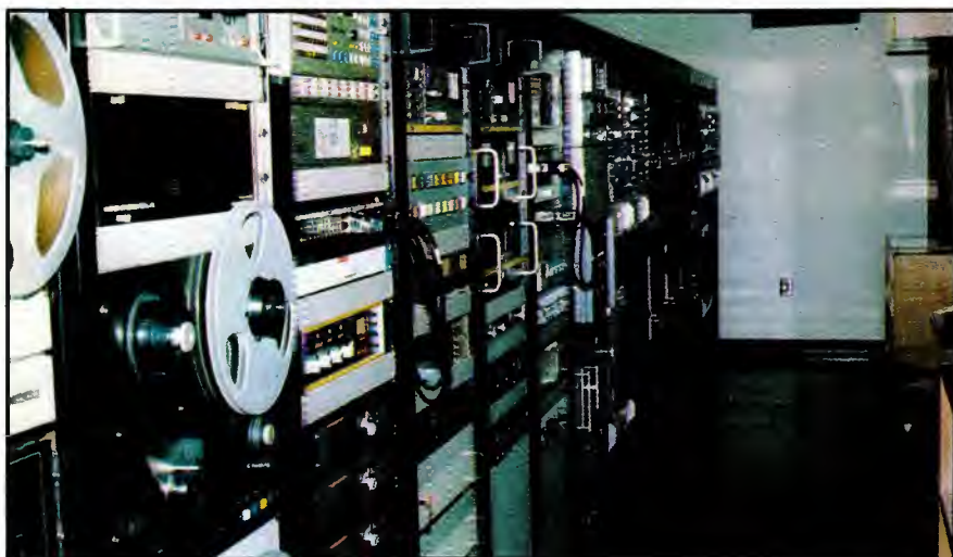
The impressive battery of equipment in the KOIT-FM automation/equipment room contains virtually all hardware needed to run the station.
