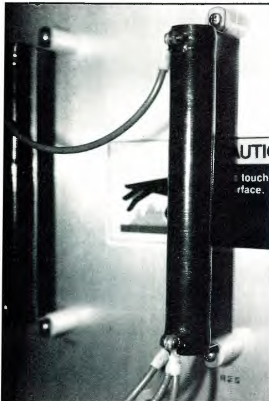
Check resistors, particularly high-power units, regularly for signs of premature wear because of excessive heating.
