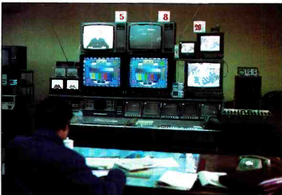
All three on-air channels can be monitored from this TV center control room in Shanghai.
