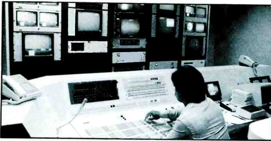
The SIN control room showing the production switcher and monitor banks.
