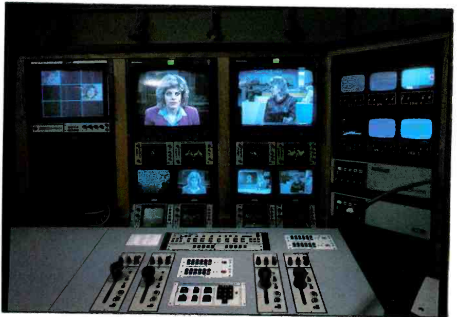
Because the cameras require no on-air maintenance attention, the crew chief's position has controls for setting up ENG feeds and graphics frames.
