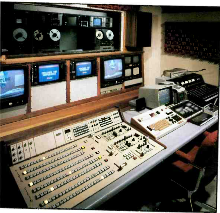
The on-line video control room of the Access Network.
