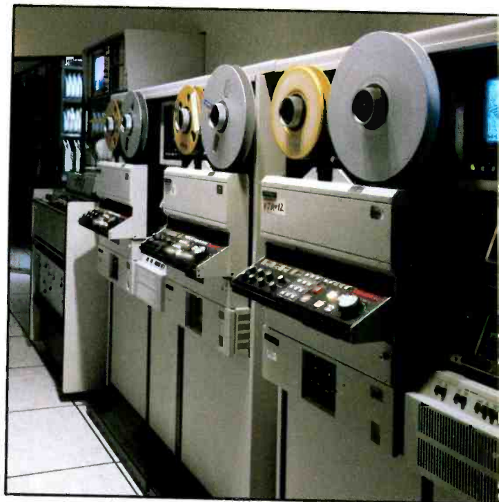
A portion of the network's master control room.
