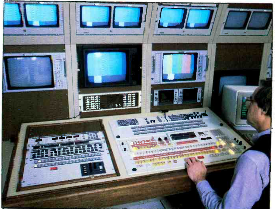
A view of the WOR master control room showing the station automation equipment and video switcher.
