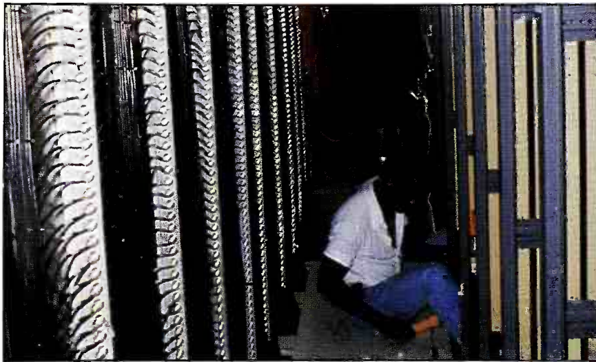
One of the 40-foot containers equipped with communications systems, audio and video patching and distribution matrices.
