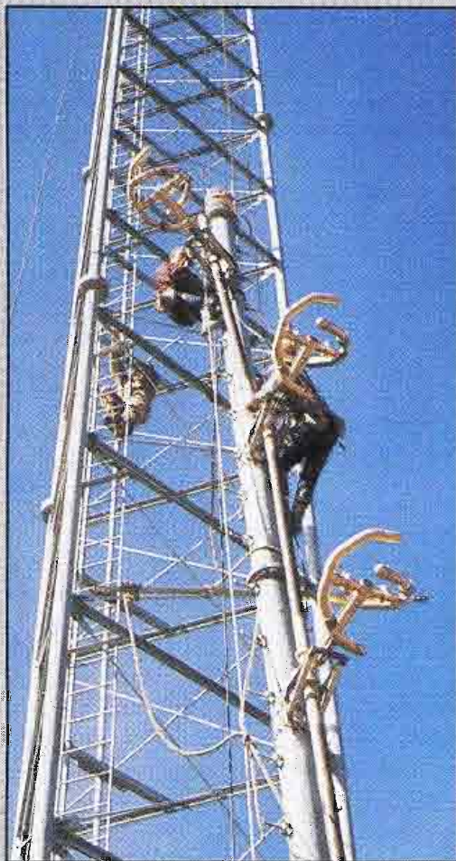
The top-mounted KLSI-FM antenna was hoisted up the tower on Feb. 7, 1987, week 24 of the project. At this point in the effort, electrical service for the transmitter building was well on the way to completion.
