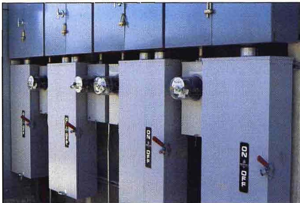
Each station in the complex has its own ac power watt-hour meter and service disconnect switch located outside the building. This switchgear and a nearby surface-mounted utility company transformer are protected from falling ice by heavy metal grating.
