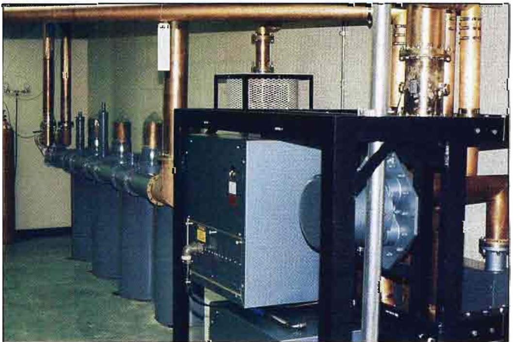
Cavity filters (shown in the background) are used on the output of each transmitter at the facility to prevent intermod problems. The combiner for the twin 25kW FM transmitters is shown in the foreground.
