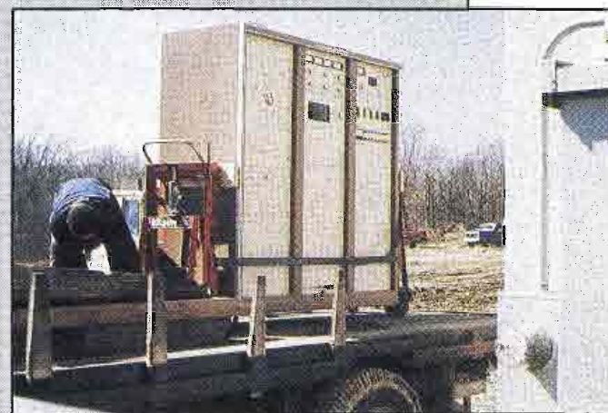
The big day finally arrived during week 28. One of the two KLSI transmitters was moved to the new site and put into service. To everyone's relief, everything worked on the first try, just as it was supposed to. The second transmitter was moved to the facility the following day.
