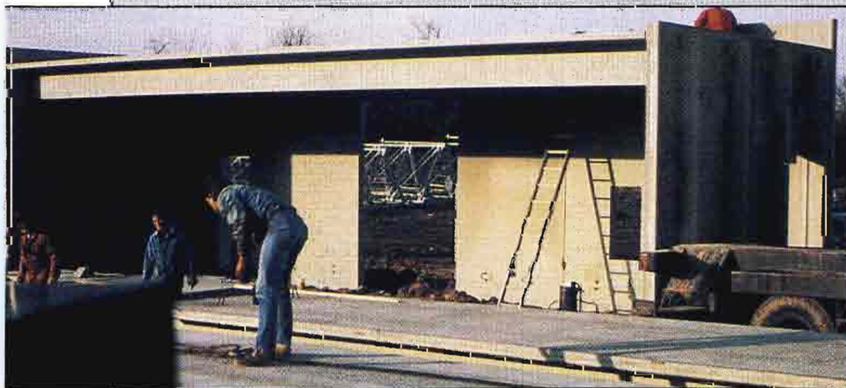
The transmitter building began to take shape during week 19 of the project. Precast wall panels were trucked to the site and lifted into place by a crane. At this point in the project, the local utility company had placed the necessary power poles and lines for ac service.
