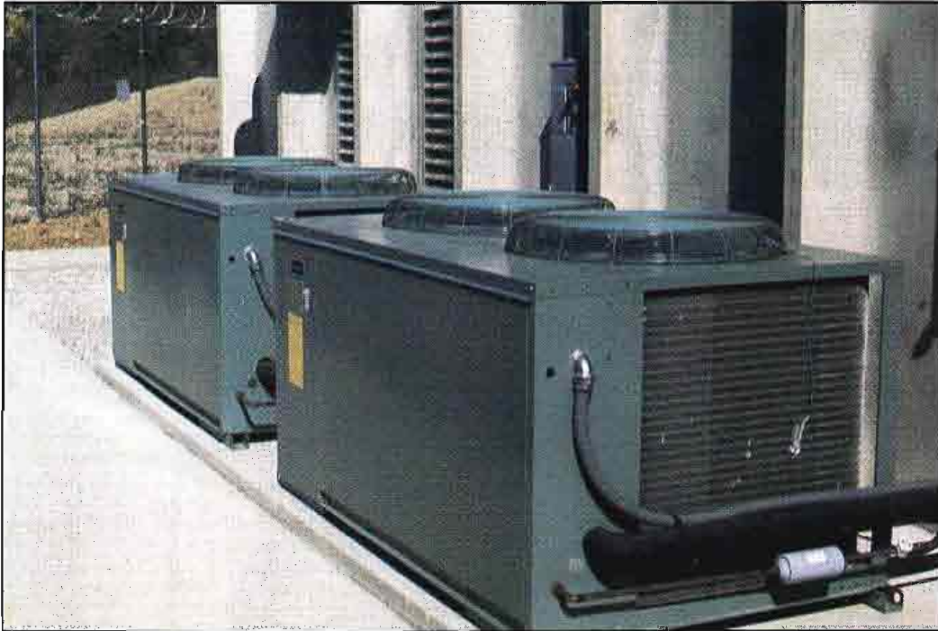
Two of the four stations have closed-loop cooling systems in which no outside air is used to cool the transmitters. Exhaust air from each transmitter is dumped into the room and large air-conditioning units are used to keep the rooms cool. The heat exchangers for one of the transmitter rooms are shown.
