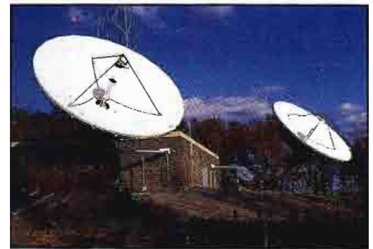
The technical center is connected via common-carrier microwave to the Bren Mar uplink site, shown here.
