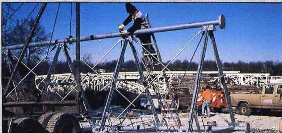
Nobody wants to put up a tower in the middle of December in the Midwest. However, KLSI didn't have a choice. The project was well under way, and it couldn't be interrupted by bad weather. Seven truckloads of steel were shipped to the tower site. Assembly of the sections on the ground began during week 15.
