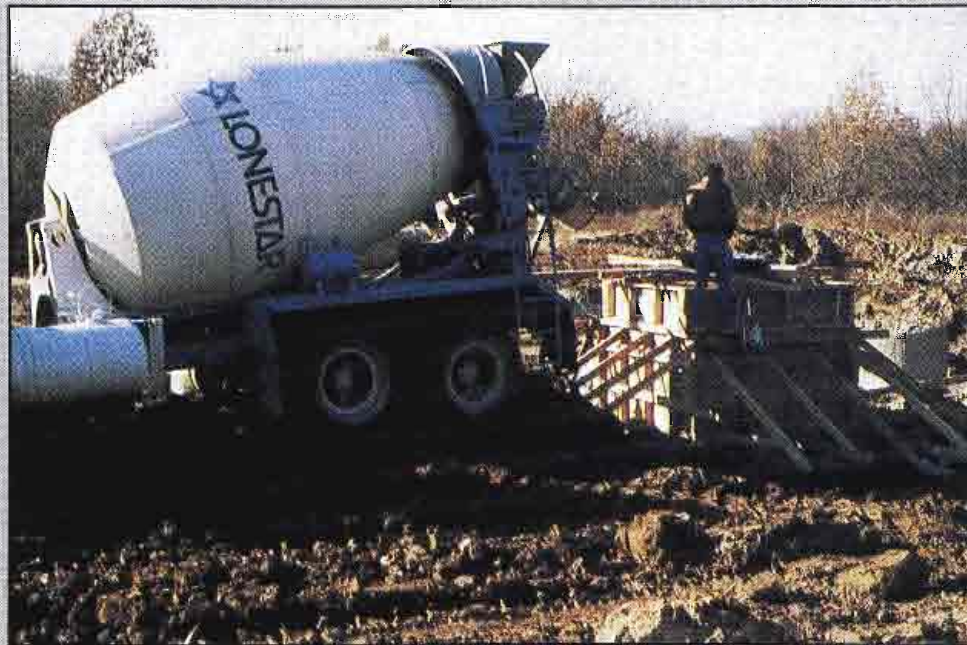
Concrete was poured at the tower base during week 12. At the same time, drilling was under way for the guy anchor posts. Some of the posts were drilled to a depth of 80 feet to ensure a sound footing and to avoid problems with the underground limestone mine.
