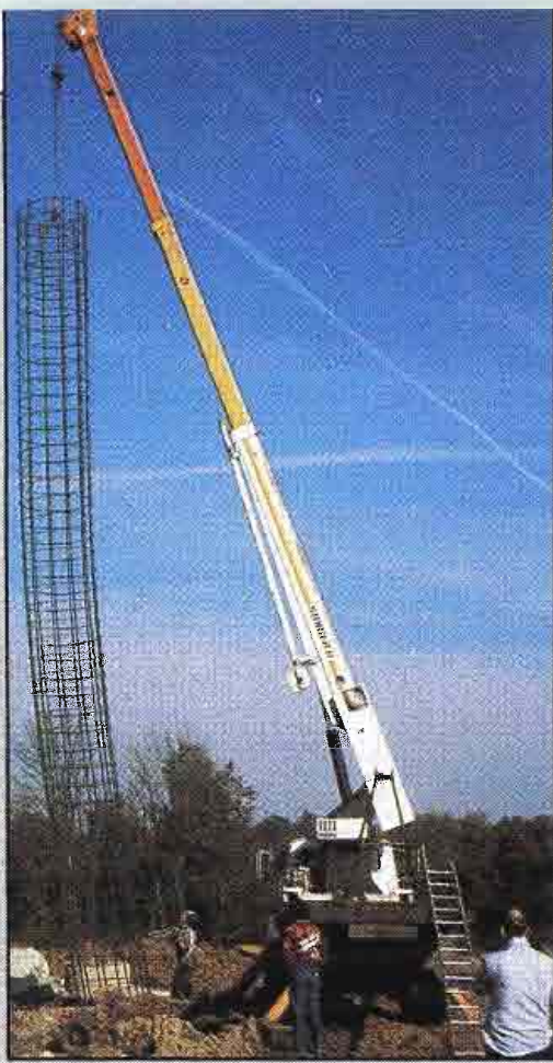
By week 10 of the project, the tower pier had been drilled and the rebar set in place. A 5-foot-diameter hole was drilled 56 feet down for the foundation of the structure.
