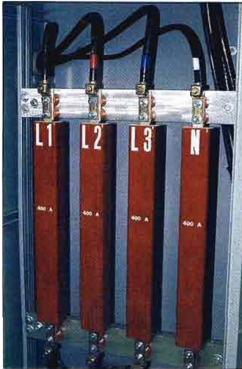
Transient protection is a major concern because of the high level of lightning activity. This transient suppressor protects the KLSI section of the facility.
