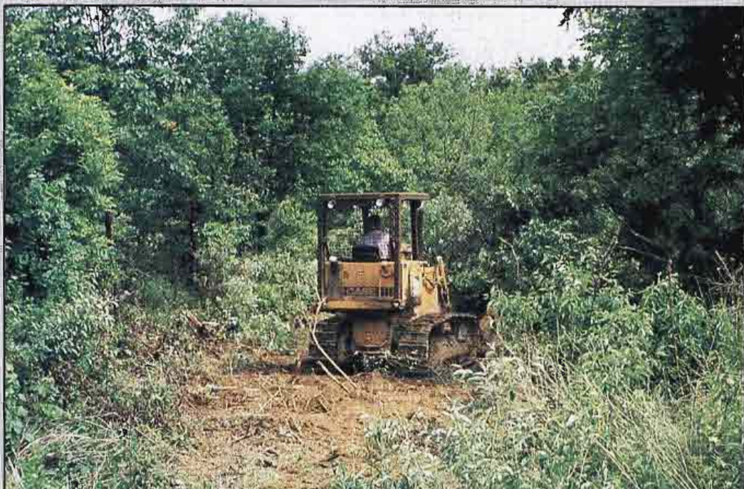
The first few weeks of the project involved clearing the land and finalizing drawings for the tower and building. A building permit was issued for the tower by the city of Kansas City, MO, on Sept. 26, 1986. (Photos by Ben Weiss.)
