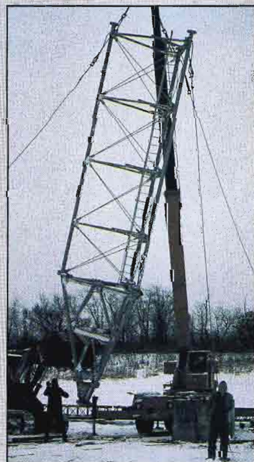
The first steel went up in the air on Jan. 10, 1987, in week 20 of the project. The base of the tower was placed, and over the course of the following six weeks, the structure slowly began to take shape. Bad weather and other problems kept the work "interesting."
