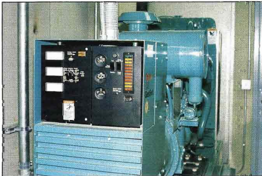
Standby power is provided only for KLSI, the landlord at the community site. Two other stations using the facility have kept their old transmitter sites for use in the event of a power failure or equipment problem.
