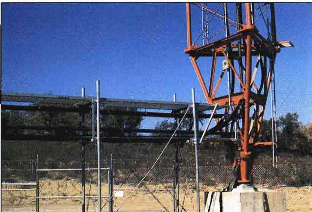
Grounding is a major concern for the transmitting tower because of the frequency and severity of lightning storms in the Kansas City area. The ground system consists of radials spread out from the base of the tower in a manner similar to an AM antenna ground. The transmission line bridge from the building to the tower can be seen below the ice shield.
